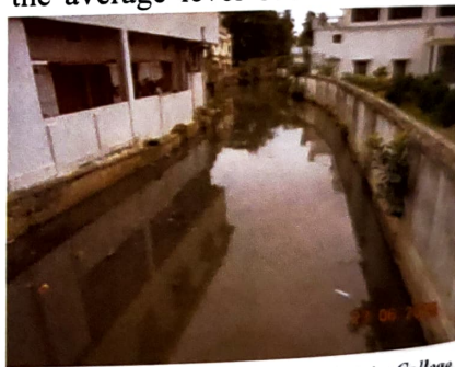
View of encroached drain near Christ College
