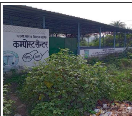
3.4.3(2) – Non-operational compost shed in dilapidated condition at Emlipara, NPP- Kanker (Dt. 19.10.2022)
