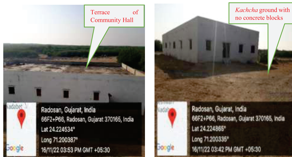
Photograph 3.1: Deficiencies in construction of Community Hall
