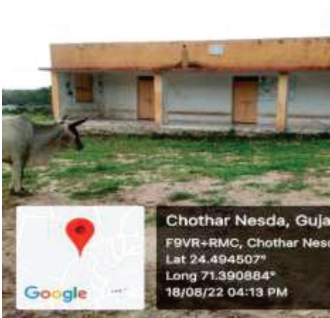
Community hall lying idle Source: Photographs taken during joint site inspection (August 2022)
