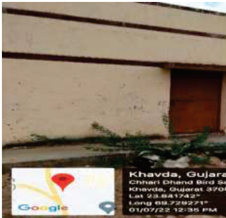
Training Centre lying idle Source: Photographs taken during joint site inspection (July 2022)
