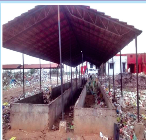
Picture 6 Non-operational VCP in Anjar NP
