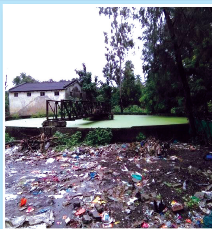
Picture 4 Untreated sewage found overflowing at non-functional STP in Valsad NP
