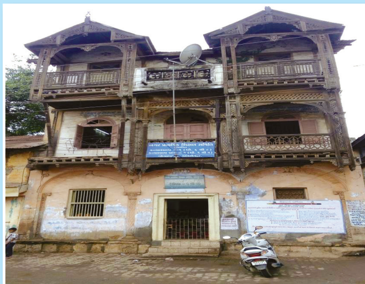
Picture 8 Kanya Shala No.1 with 350 students functioning in dilapidated residential building
