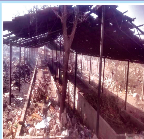
Picture 7 Dilapidated VCP in Surendranagar NP
