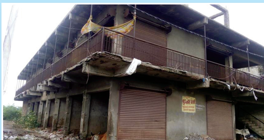
Picture 2 Dilapidated condition of a shopping complex at Pakshi Bhavan in Bavla NP
