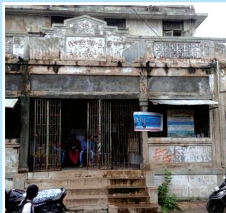
Picture 10 Dilapidated building of Maternity Home in Ankleshwar NP
