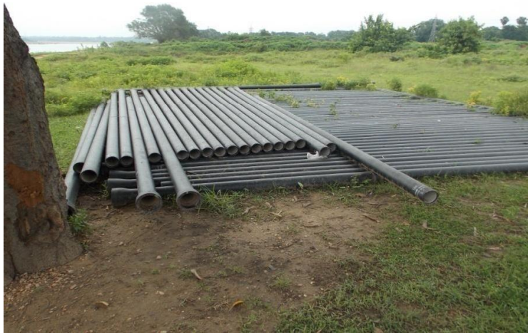
Figure :Kulti municipality pipes stacked without security
