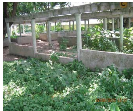
Dilapidated Vermicompost plant of model facility
