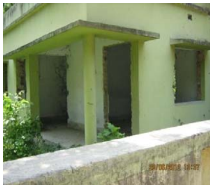
Dilapidated building of model facility
