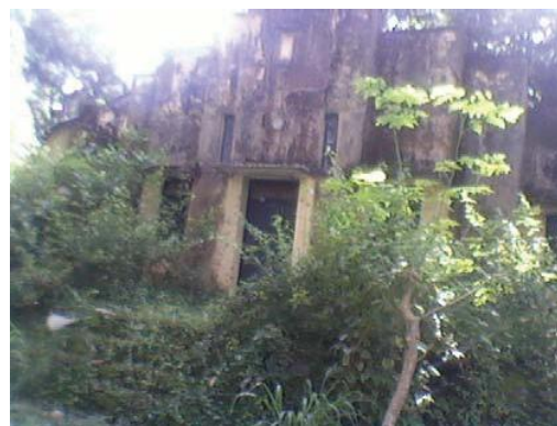
SISI building in dilapidated condition
