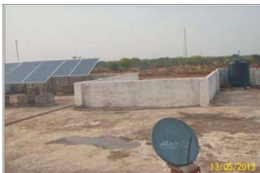
Photograph showing Solar system at Boys Hostel at Borsi block-Kasdol.
