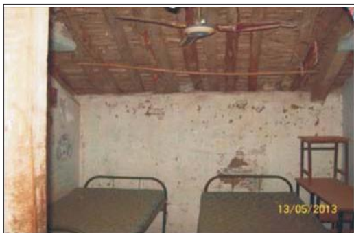
Photograph showing deteriorated rented building of Girls Hostel, at Kasdol.
