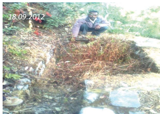
Non-functional Sarna Canal
