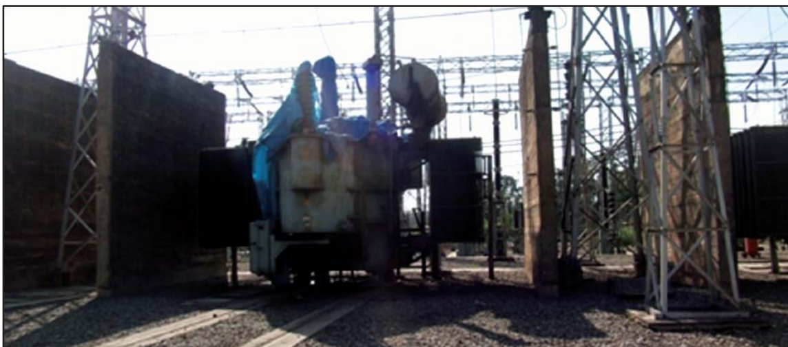
Damaged power transformer at Grid sub-station Udhampur
