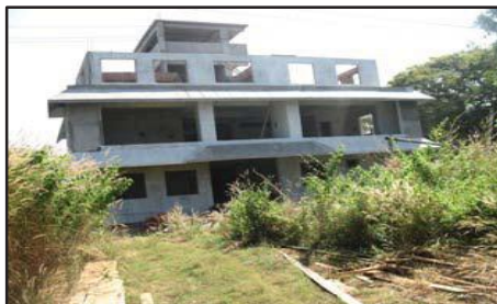
Incomplete CPS at Azheekal
