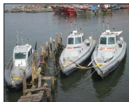
Damaged/make shift jetty at Thottappally
