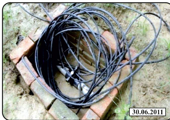
Drip system in Jaunpur
