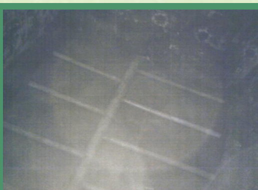
Rapid sand filter chamber without filter media
